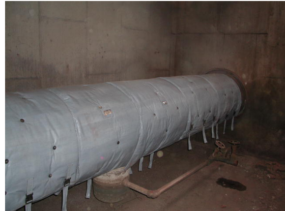
Double Slip Expansion joint & Piping
