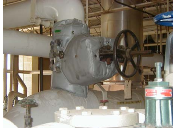
8" 250# Gate Valve – 150 psi Steam Header
