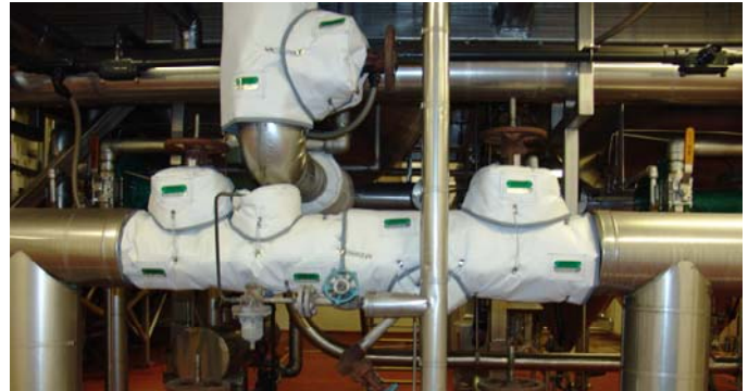
Control Valve Station
