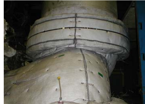
Multi-Stage Steam Turbine
